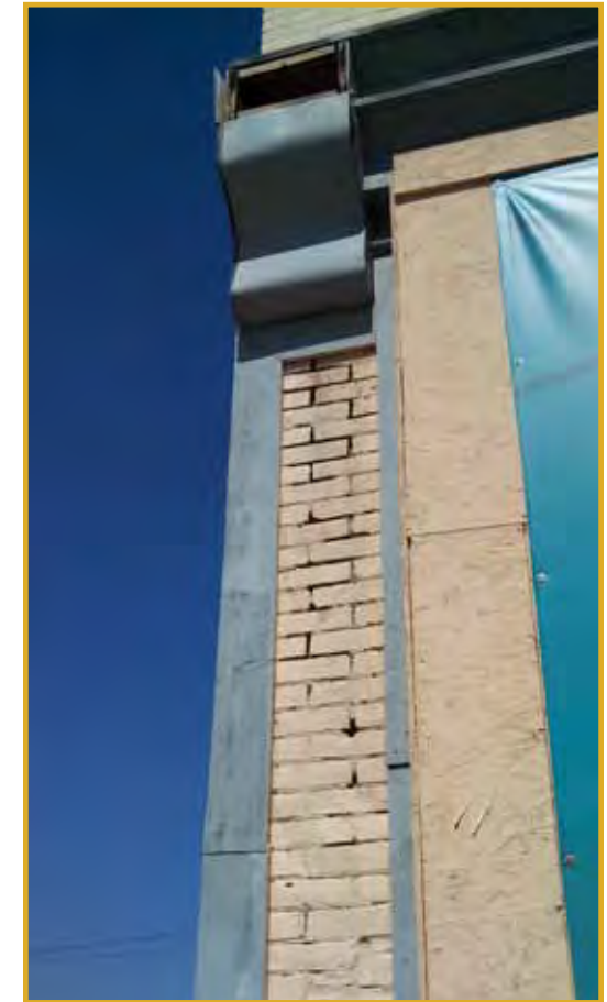
Above: Deteriorated mortar joint
