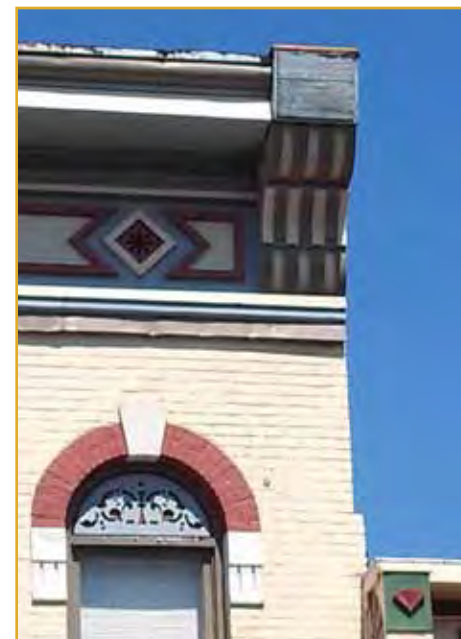
Above: Metal component damage
